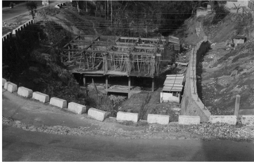
Figure 12. Building construction in progress in the down stream of the natural drain of Figure 11, near Bank Tinali, Itanagar, March 2004.
