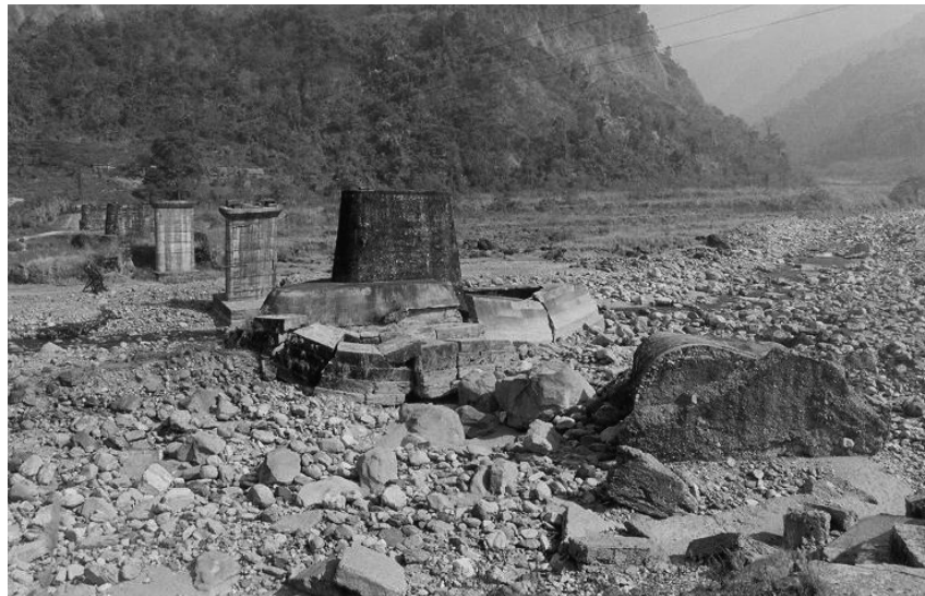
Figure 14. A collapsed bridge over Deo Pani River near Roing, Lower Dibang Valley District, Arunachal Pradesh, February 1999.
