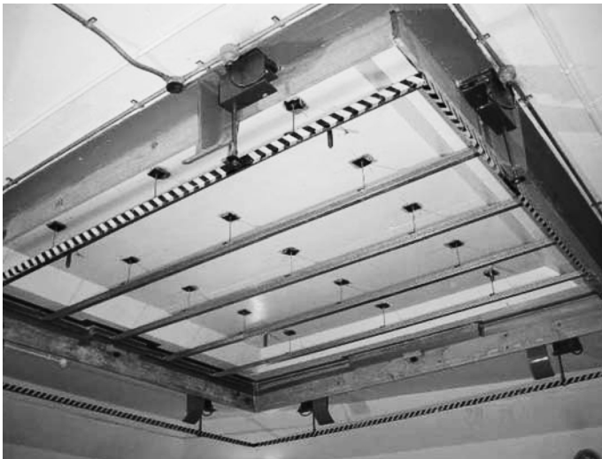
Figure 7. Array of battens suspended from a concrete floor before the installation of the ceiling panel.
